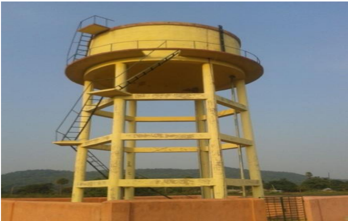
Piped water overhead tank to village Nuadihi of Reamal block
